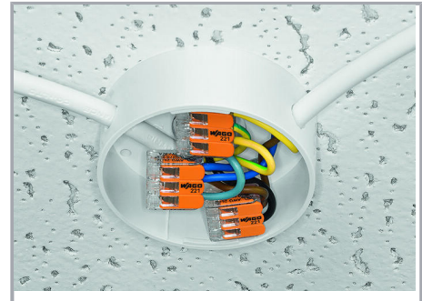
Lighting distribution in a ceiling canopy
